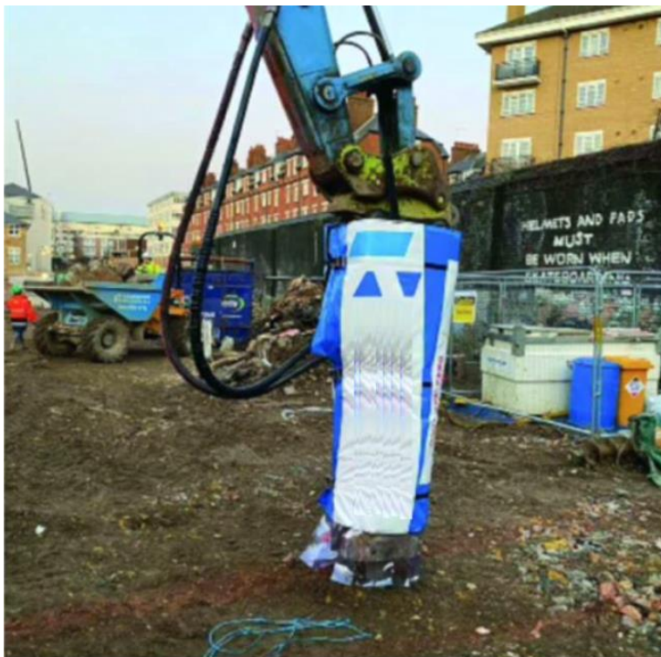
Figure 2 Example Acoustic Shroud Around Breaker
